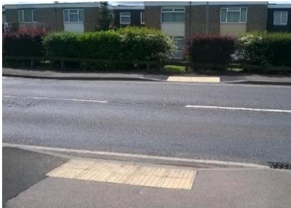
Figure 1 Example of a dropped kerb
